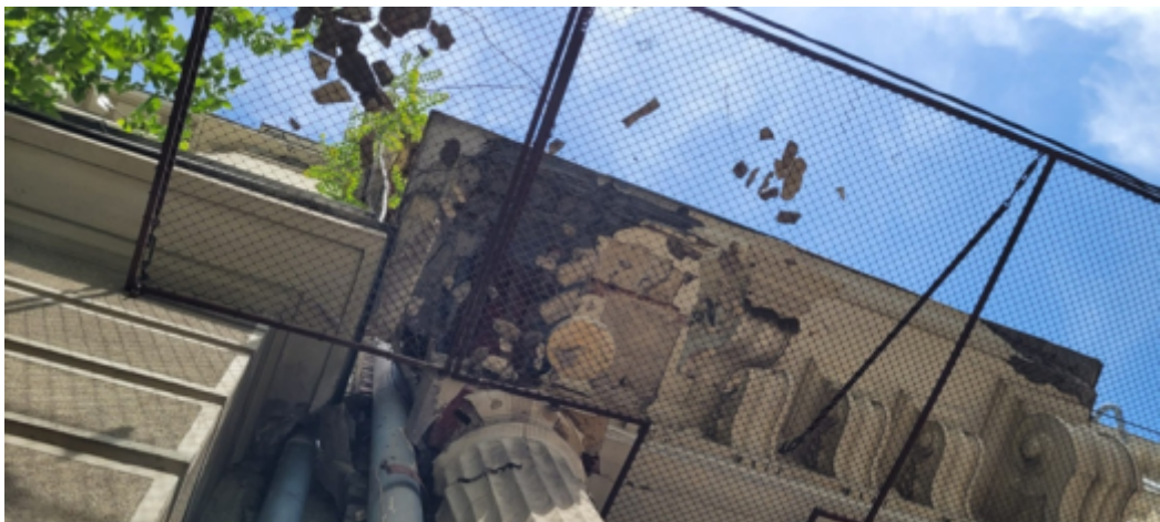
A Crumbling Building With a Protective Mesh
